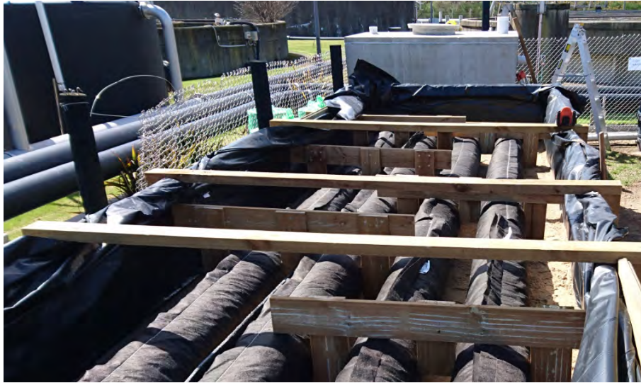
Photo 2. Distribution box during installation showing the two outlet ports at each side
